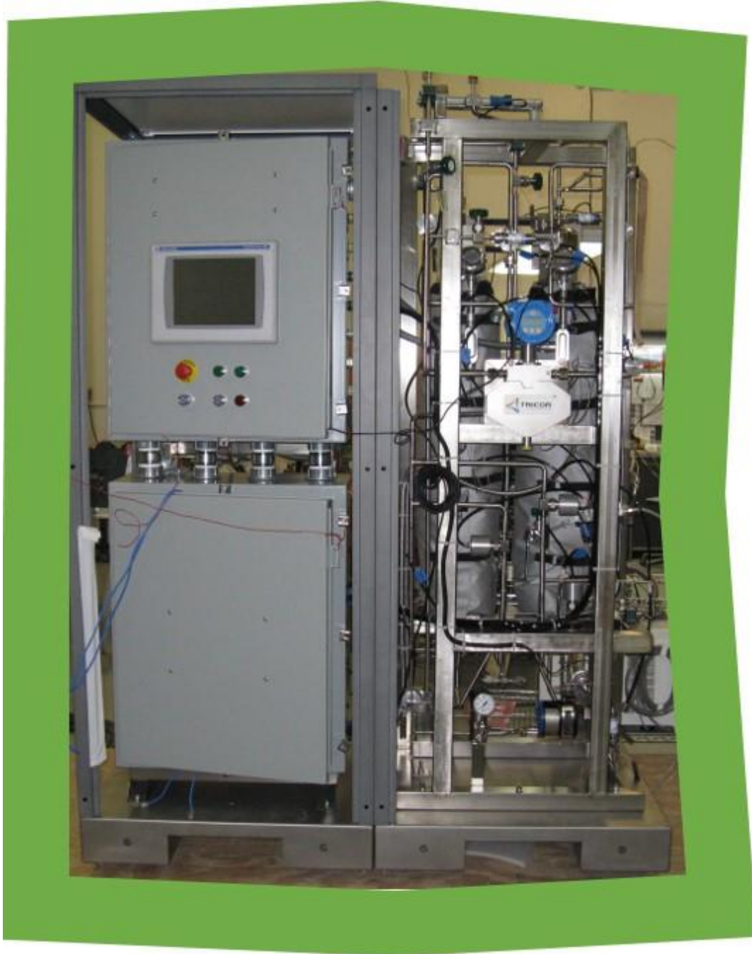
The sub-frame with vessels and plumbing (at right) installed on the 60"W x 30"D base made easy by a removable enclosure frame.
